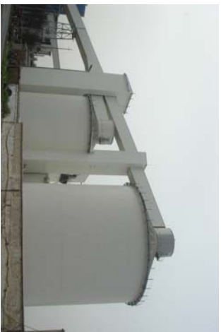
Fig. 5: New conditioning and storage silos
